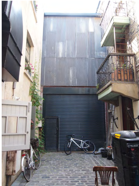
External elevation of Building taken from Peck's Yard. External boundary made up of profiled metal sheeting
